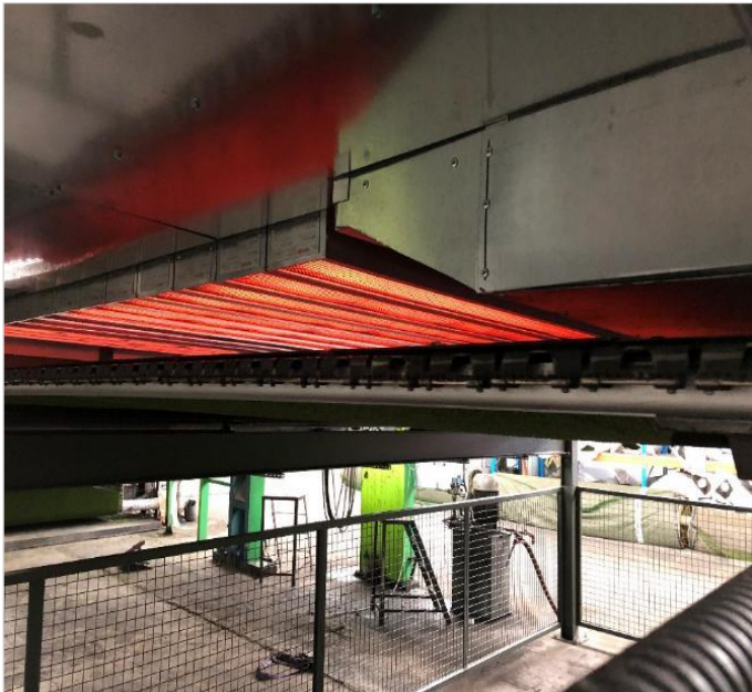
→ Roof-mounted electric infrared heating panels
