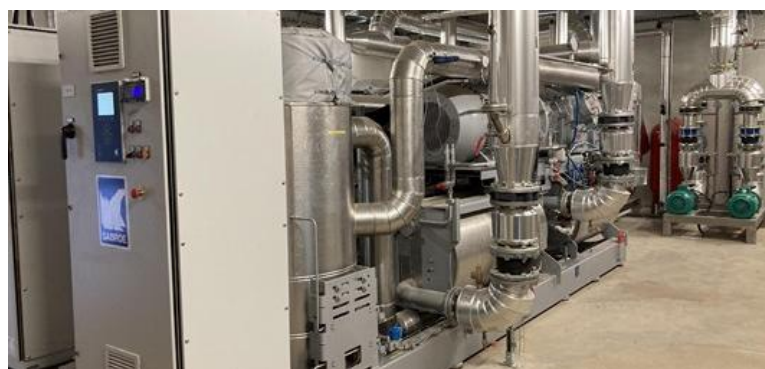
→ View of the two-stage heat pump
