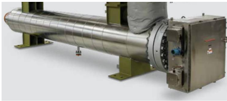
→ Electric heater installed
