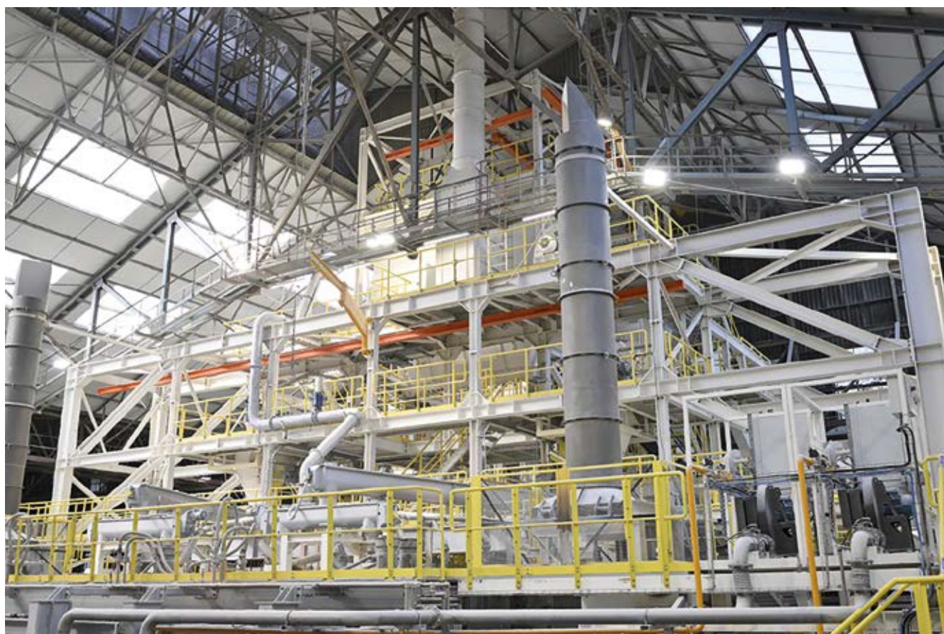
→ 100% electric glass furnace, Cognac © Verallia
