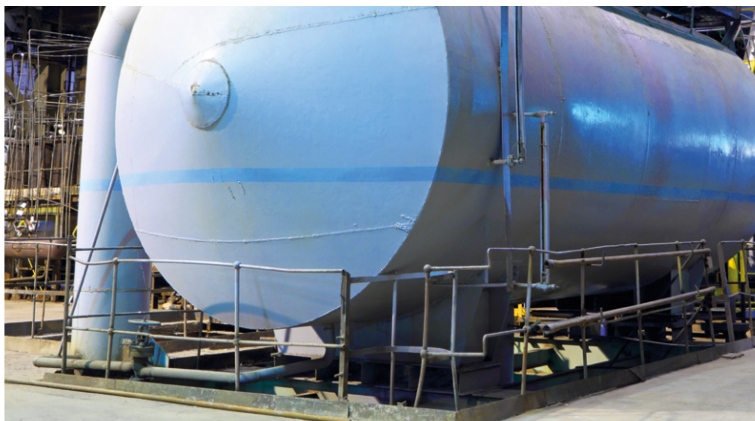
→ Indoor tank in a petrochemical planta © hramovnick/Shutterstock
