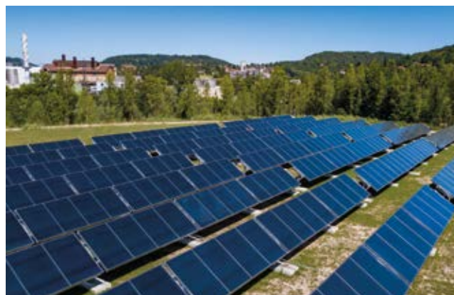
→ Thermal-solar installation powering the Condat papermill (LECTA group) © Newheat
